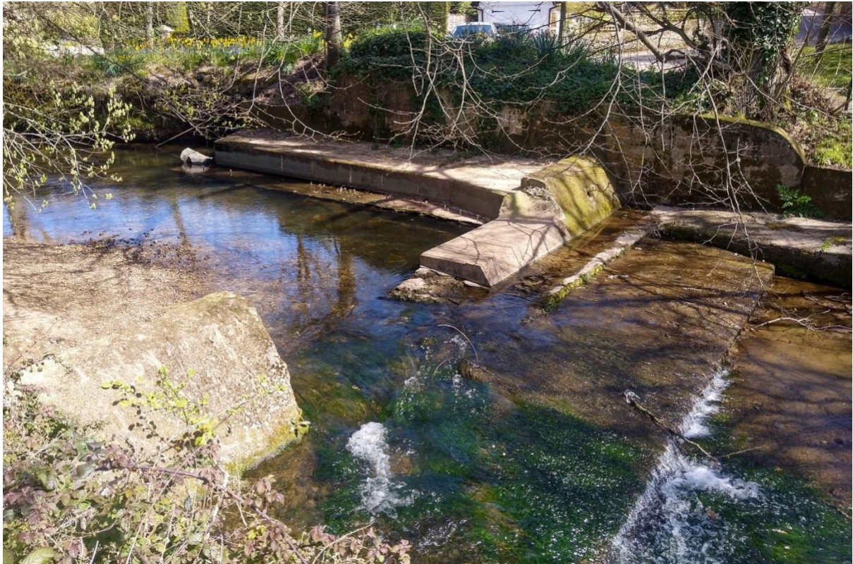
Figure 17 Another old weir that has had a section removed. Despite this improvement for fish passage, the three shallow steps downstream are a significant impediment to fish passage. Total removal would be the best course of action. SY 12969 88498
