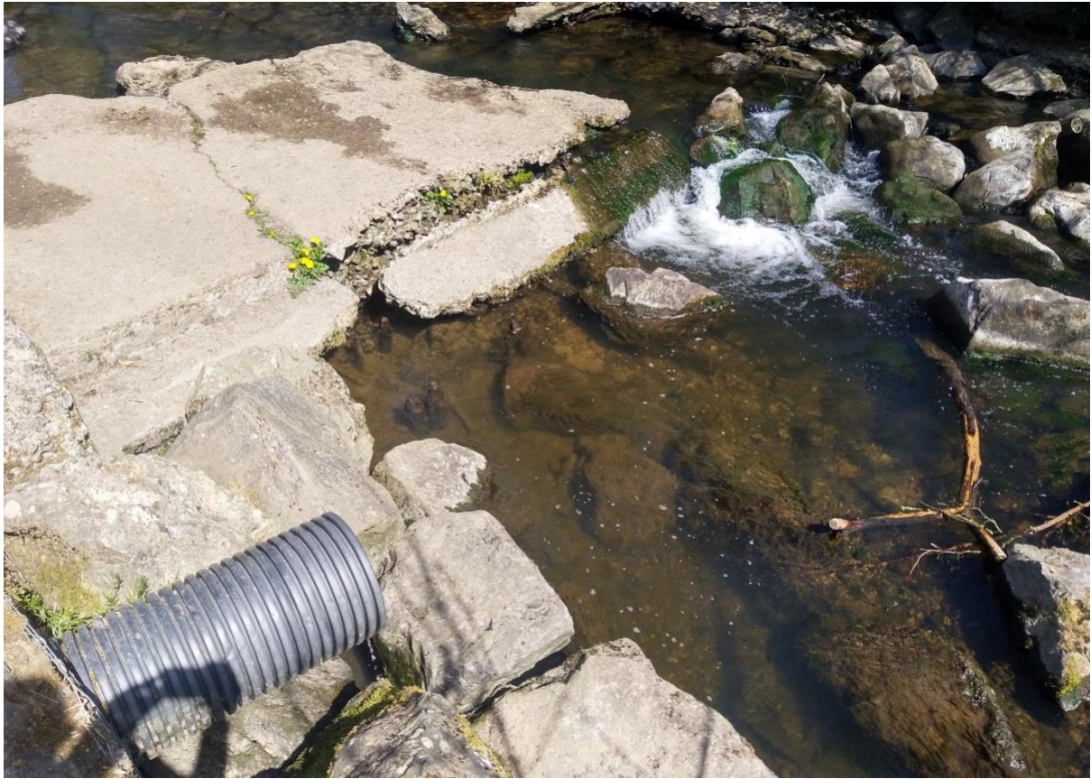
Figure 15 Sewer Storm Overflow Permit No: 201828 no spill duration monitoring available. Algal growth suggesting excessive nutrients in this area. SY 12956 88575
