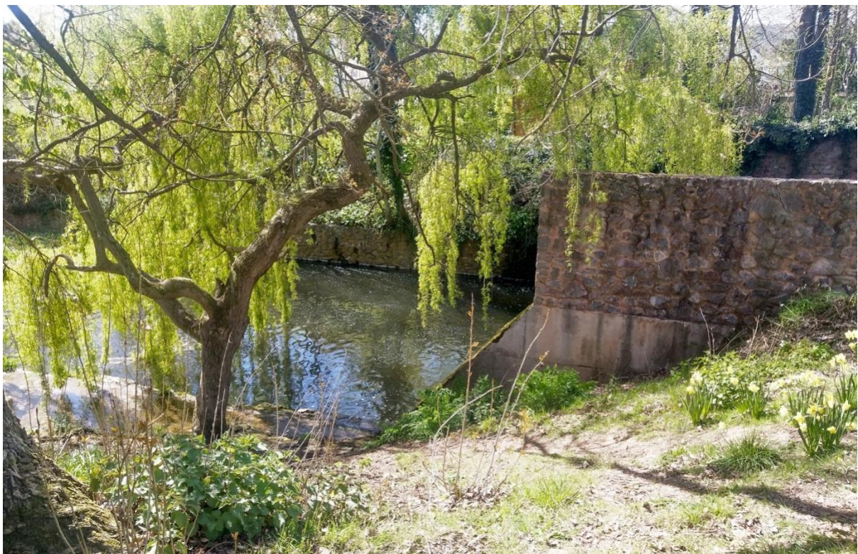
Figure 28 The LB retaining wing wall of the School Weir seen from the top of the bund (Figure 27). SY 12790 87895
