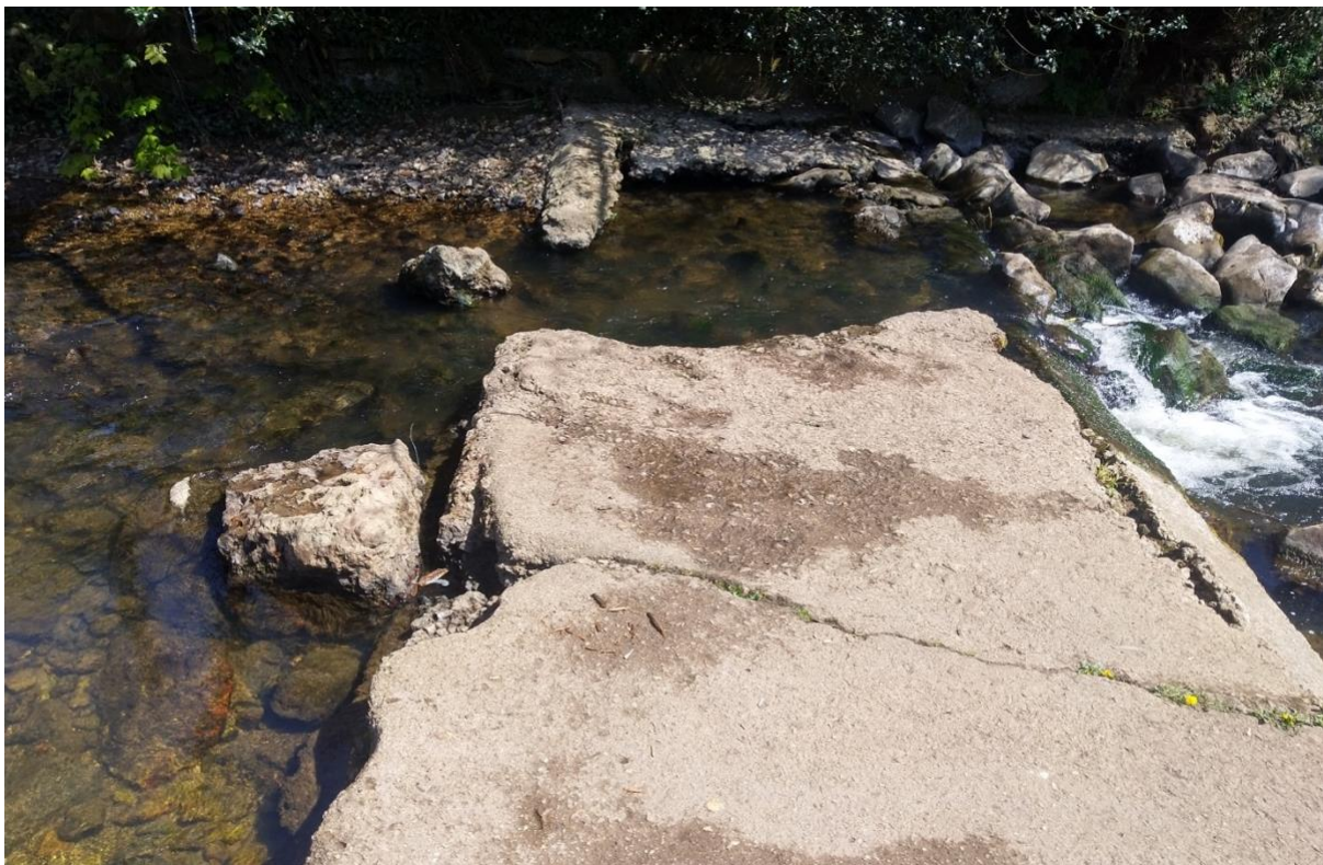
Figure 14 The remains of an old weir structure. Despite the breach, it is impounding the reach above and could be entirely removed. SY 12956 88575
