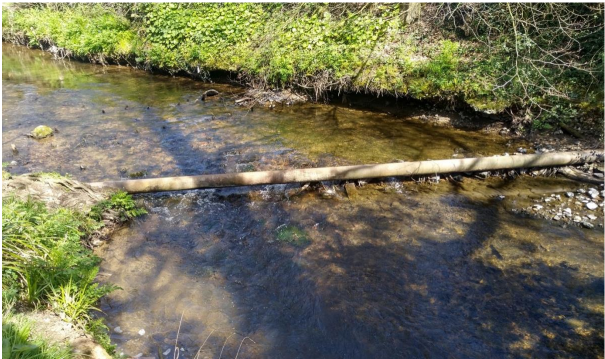
Figure 16 A sewerage pipe crosses the river. With high flow velocities common, this is vulnerable to fracture by passing debris. The asset owner is liable for the environmental damage such a fracture will undoubtedly cause downstream. Liaison with the owner to find a re-routing solution is advised. SY 12977 88539
