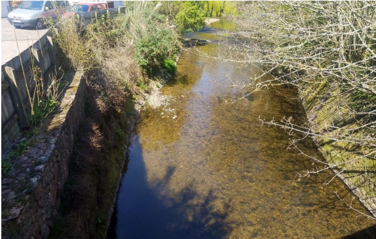
Figure 29 Looking upstream from Salcombe Rd Bridge. The hard engineered channel and reduced sediment load have contributed to a uniform and featureless channel. In combination with river and weir improvements upstream, low lying large woody material (LWM) could bring back some habitat diversity without affecting high flow conveyance. SY 12781 87811
