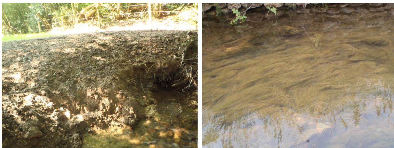
Left: One of many areas of cattle poaching (trampling) on the banks of the River Sid.
