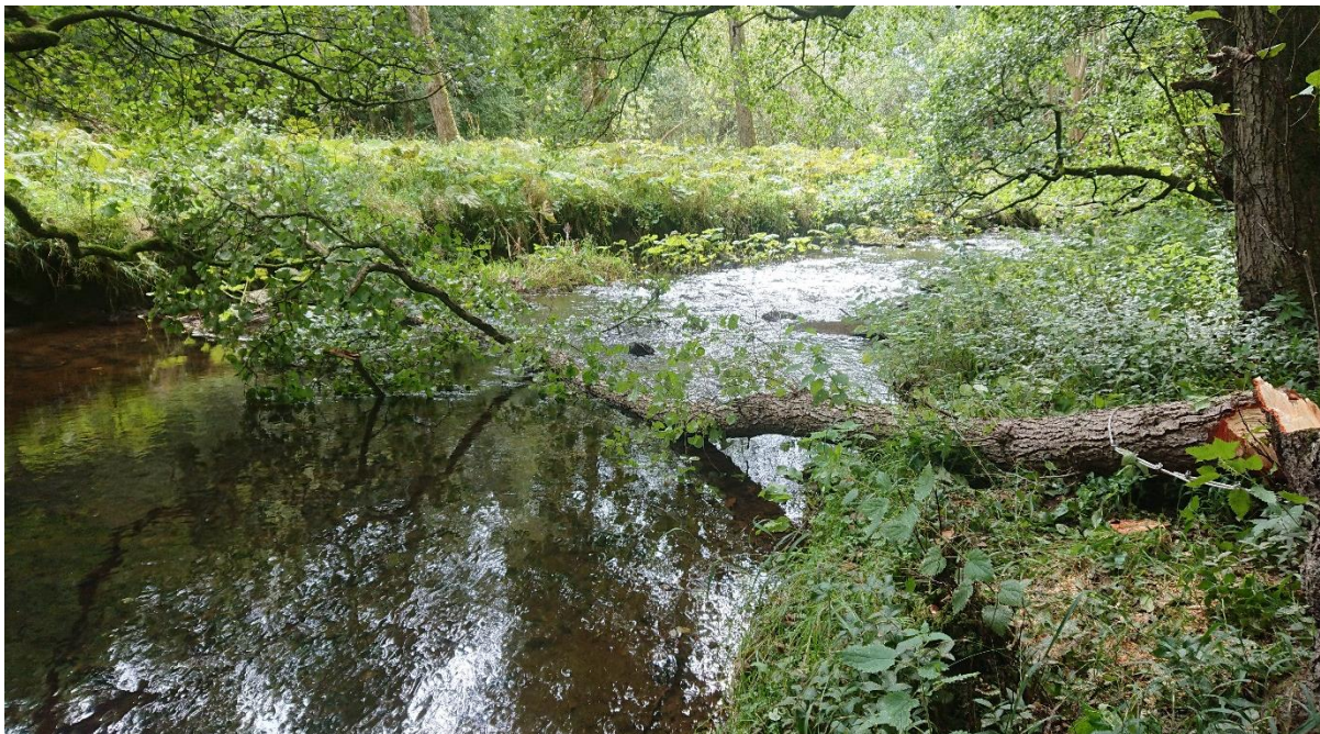
Figure 9: An example of an alder tree kicker on the Flasby Beck, with steel rope used to secure the felled tree to its stump.
