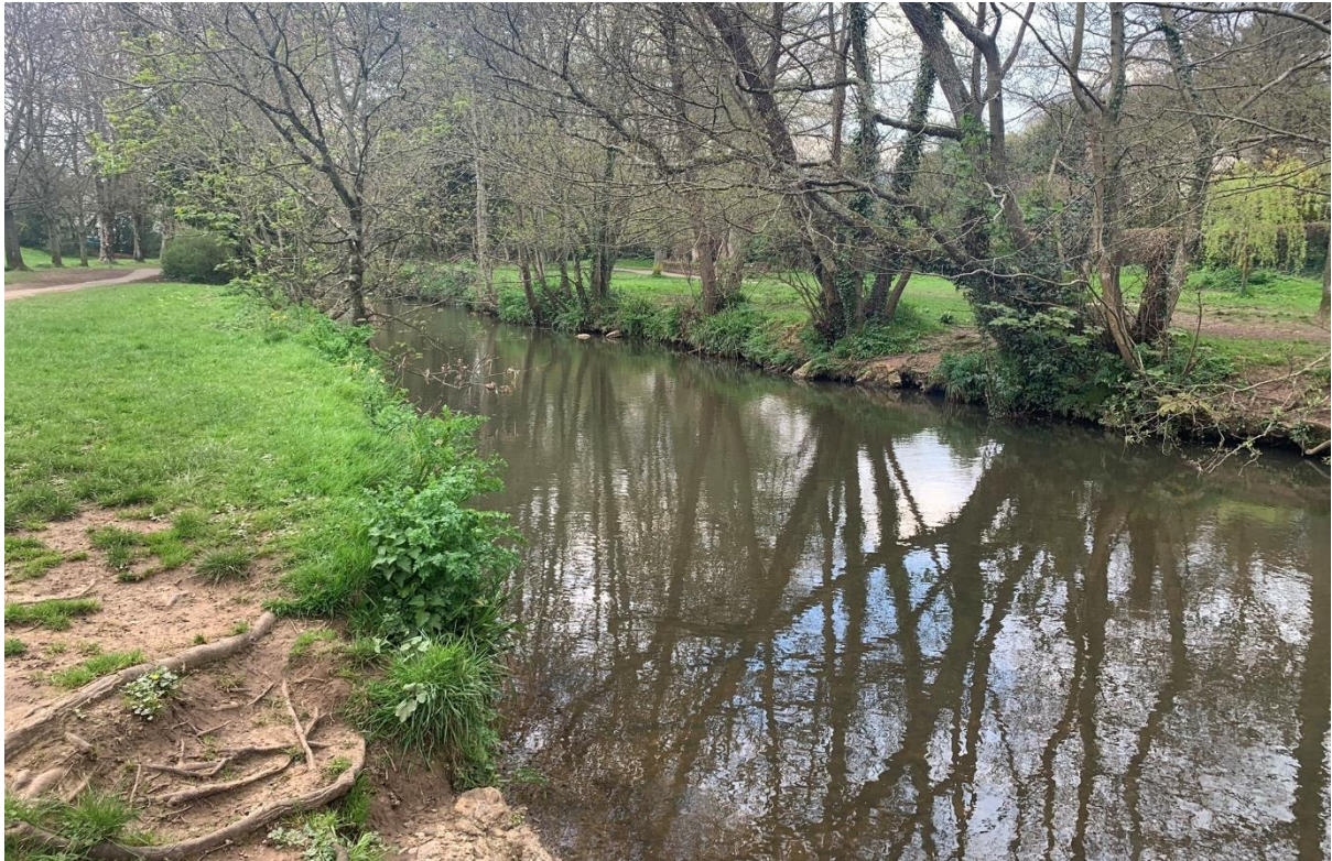
Figure 7: The River Sid towards the downstream extent of the reach inspected. Again, uniformly straight and lacking physical diversity and habitat.
